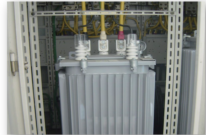
High efficiency transformer at the Mie plant
