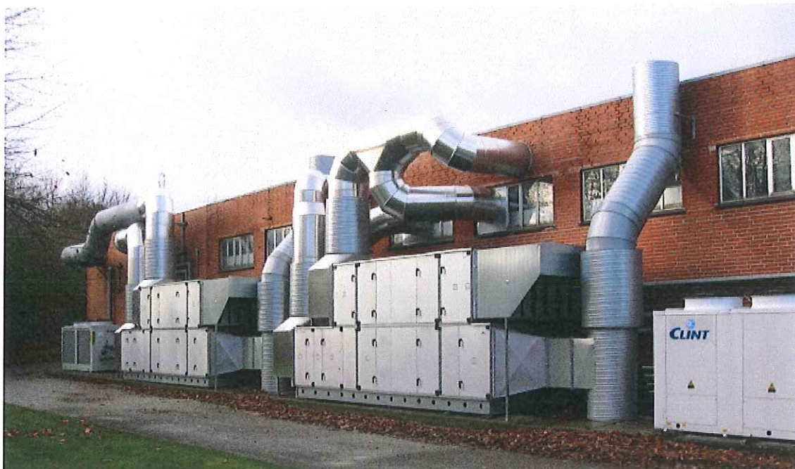
Ventilation and cooling system
