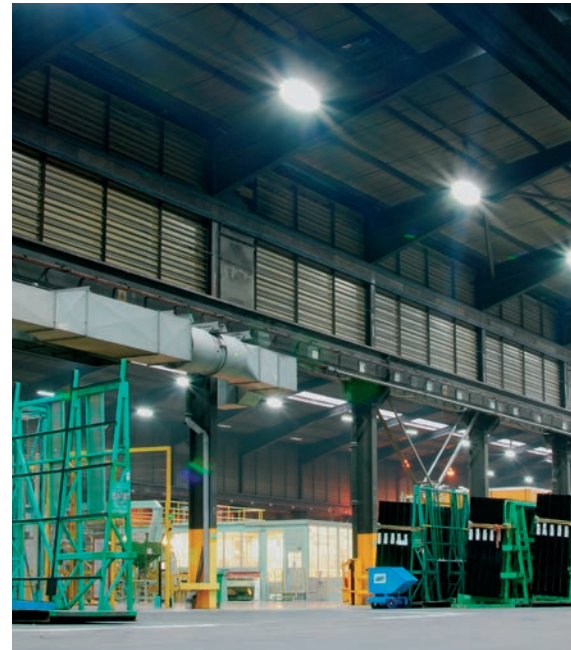
Recently installed factory lighting is on PIRs which dim automatically when the natural lighting reaches an acceptable level
