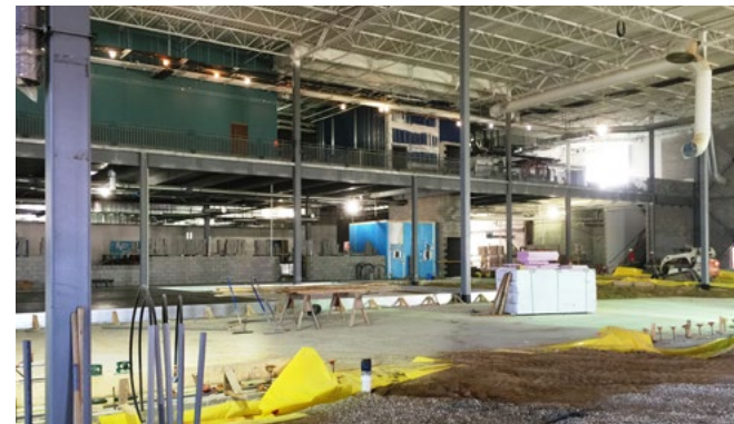
Construction of a processing center that will house customer service, logistics and operations began in 2014.
