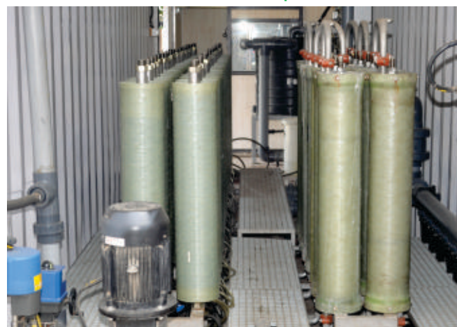
Containerised Reverse Osmosis Plant for re-cycling of treated effluent at Car Plant, Pune
