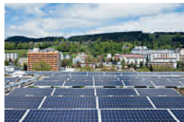
TAG Heuer's photovoltaic installation at La Chaux-de-Fonds.
