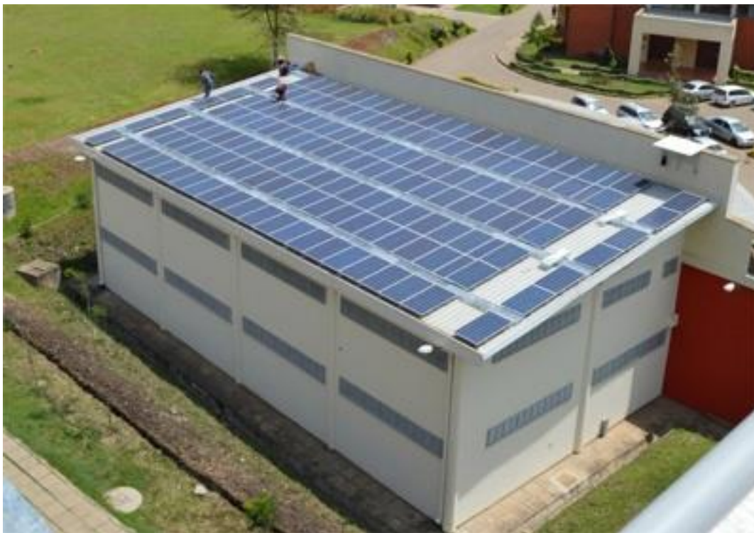
Figure 3: Solar roof: Solar panels installed on Strathmore Law School building (40kW)
