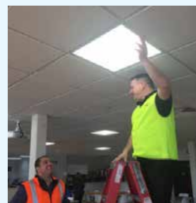
Engineering Manager at Aspen's Dandenong site inspecting the newly installed LED light
