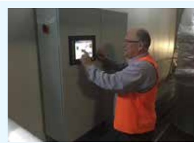
Facilities Manager of Aspen Dandenong operating the new Supervisory Control and Data Acquisition (SCADA) system
