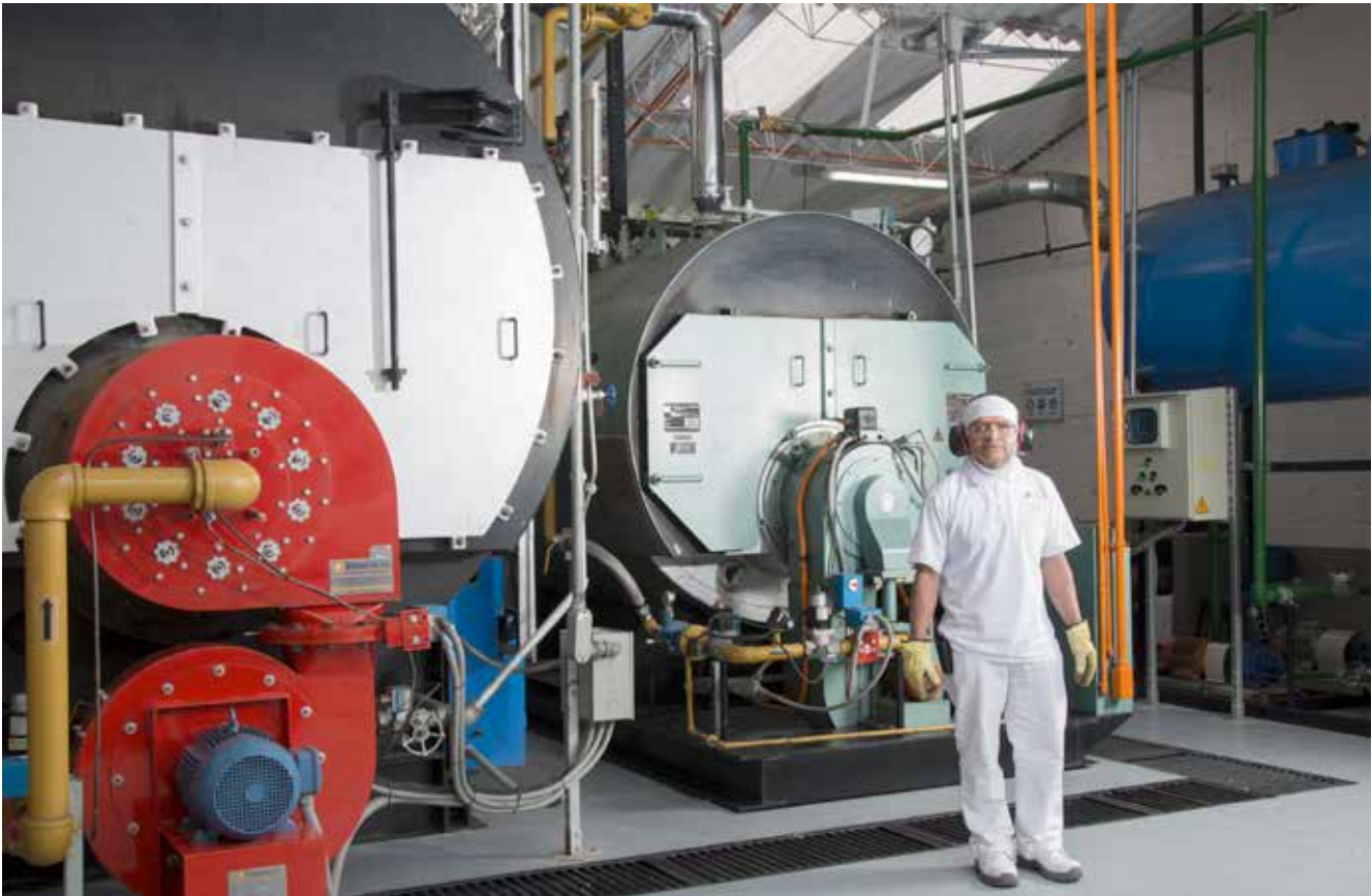
Boiler operator at the Cold Cuts Business plant in Bello, Antioquia.
