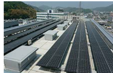
Solar panels installed on the roof of the headquarters building
