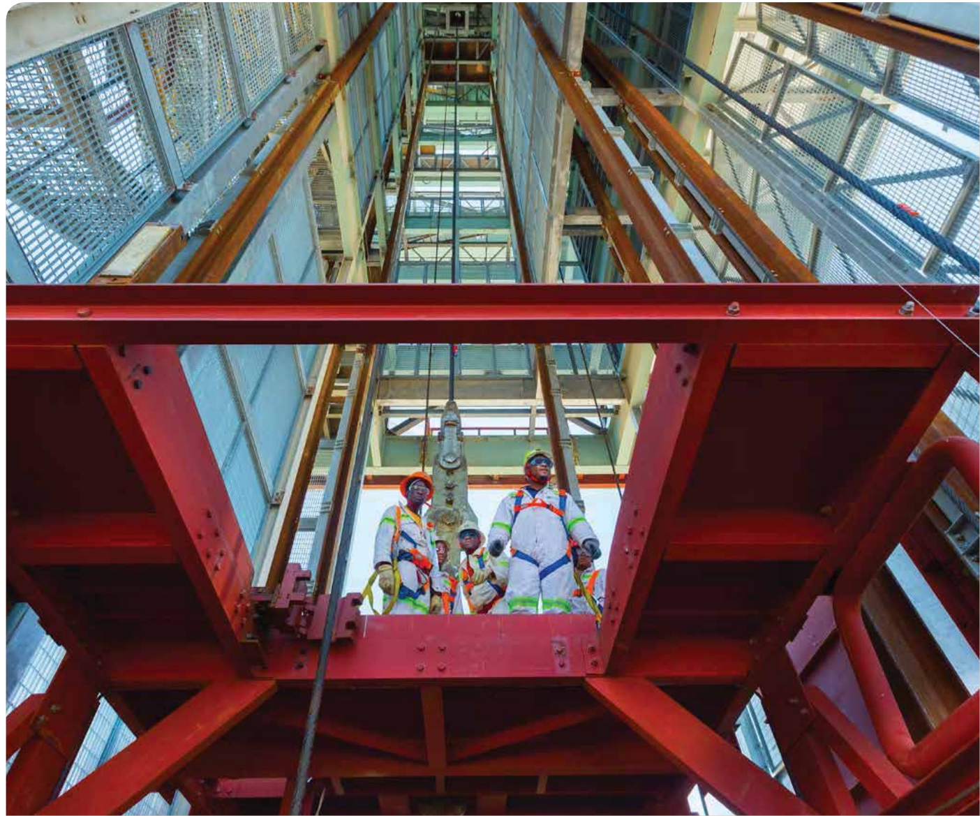
↘ The equipping skeleton, which is being used to equip the Main shaft at Styldrift I
