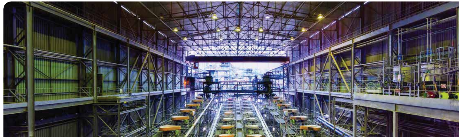
↙ A view of the concentrator flotation and cleaner circuits
