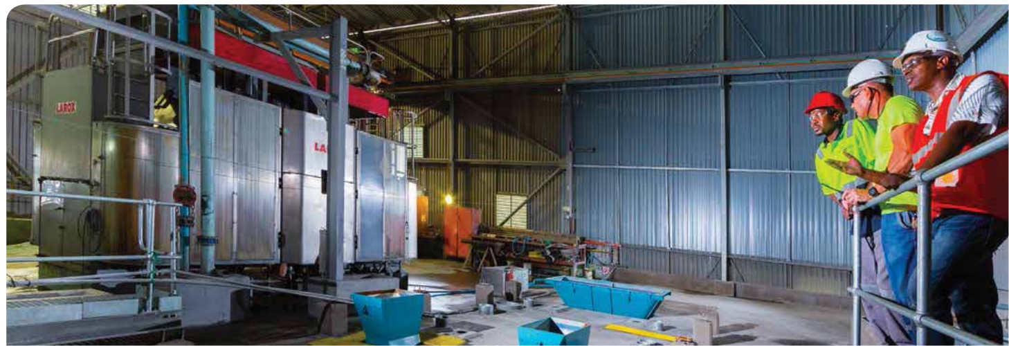
The installation of the new Outotec Larox® filter, which is part of the expansion of the RBPlat concentrator, in progress
