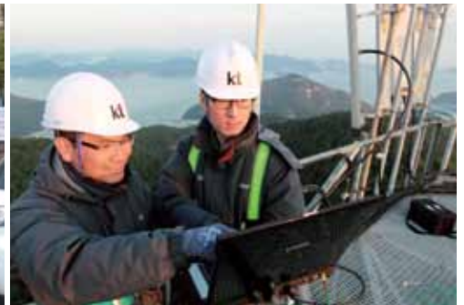
Expanding transmitting and receiving stations for vessel wireless communications
