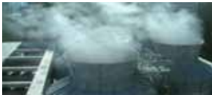
Counter Flow Tower/Open Cooling Tower
