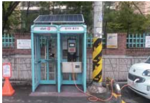
Utilizing public telephone booth as a charge station for electric vehicles
