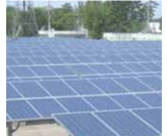
Gangneung PV Plant
