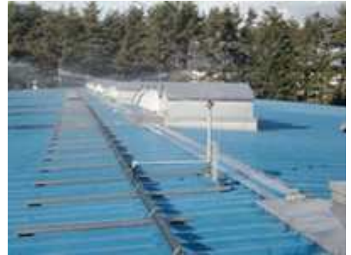
Running status of circulating roof spray system
