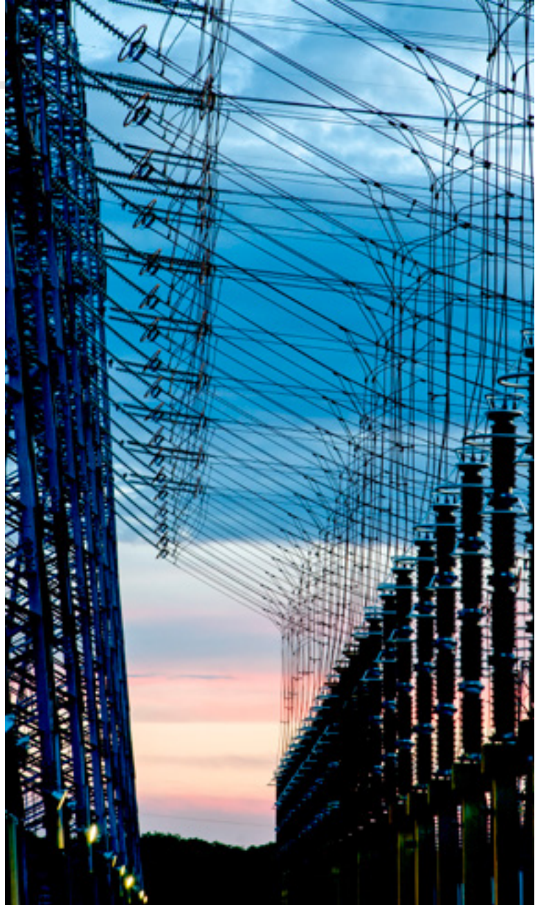
HPP MARIMBONDO SUBSTATION (MG/SP)
