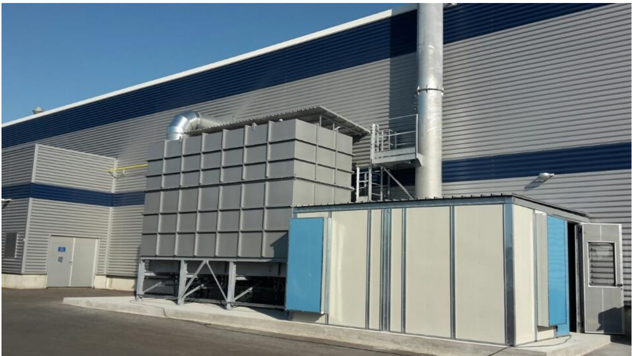
Regenerative Thermal Oxidizer Plant
