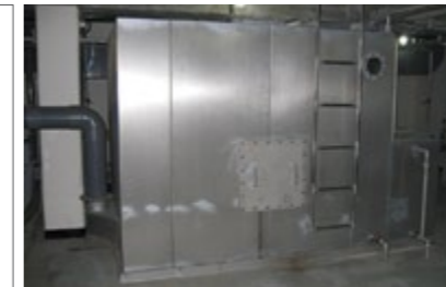
Odor Control Technology Facility
