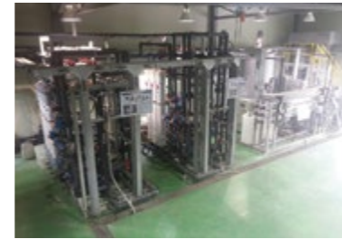
Intelligent Membrane Water Treatment Pilot Plant (Daegu)
