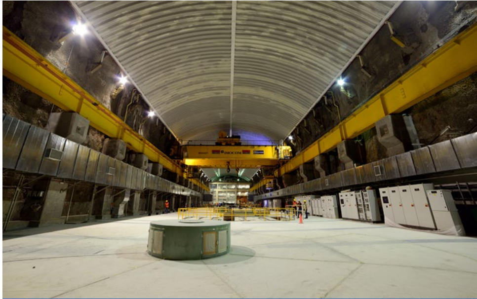
Machine station. Sogamoso Hydroelectric Power Plant.
