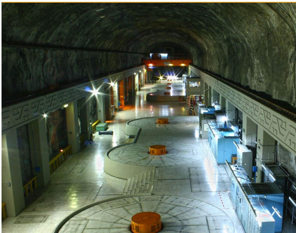
Machine station. San Carlos Hydroelectric Power Plant.
