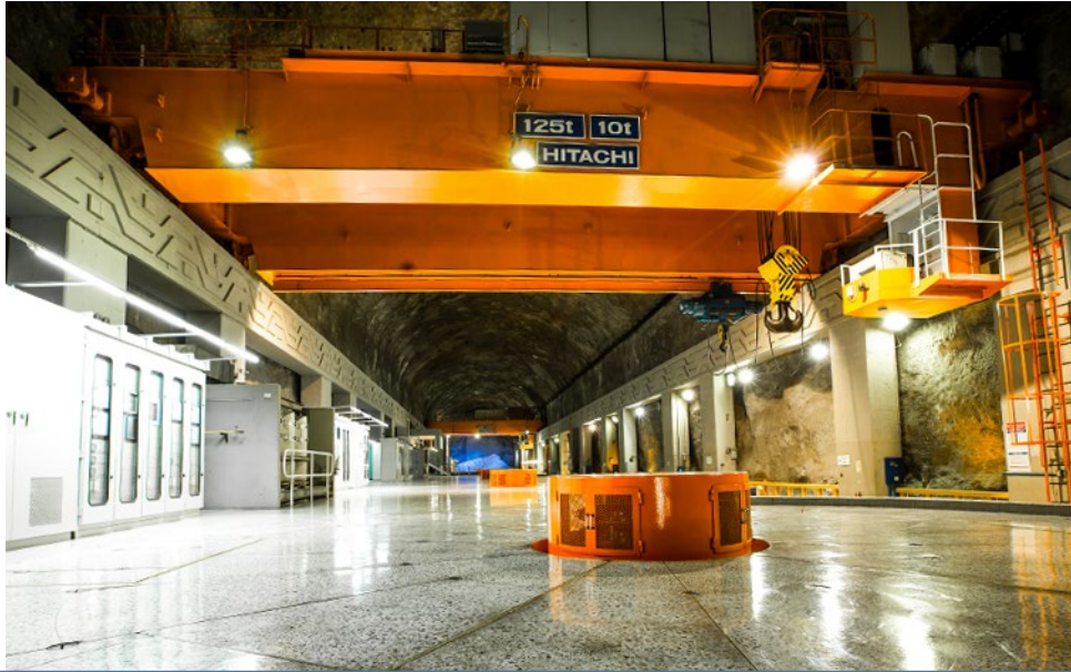
Machine station. San Carlos Hydroelectric Power Plant.
