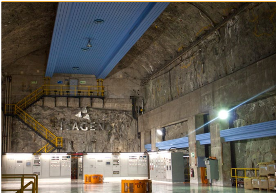
Machine station. Jaguas Hydroelectric Power Plant.
