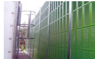
A soundproof wall around the cooler
