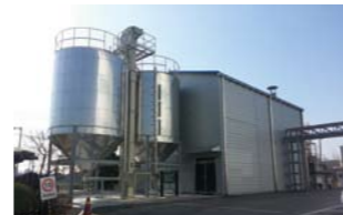
A wood pallet boiler at the Eumseong tofu plant
