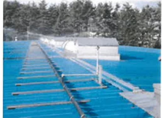
Running status of circulating roof spray system
