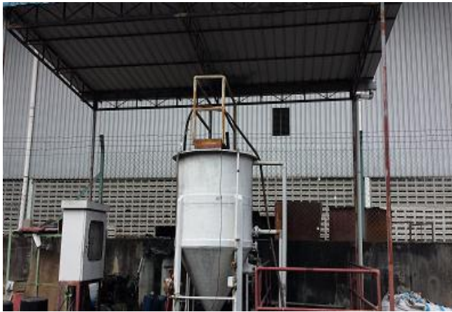
Ink Treatment Plant
