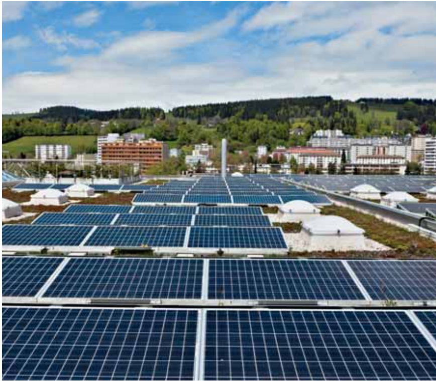
TAG Heuer's photovoltaic installation at La Chaux-de-Fonds.
