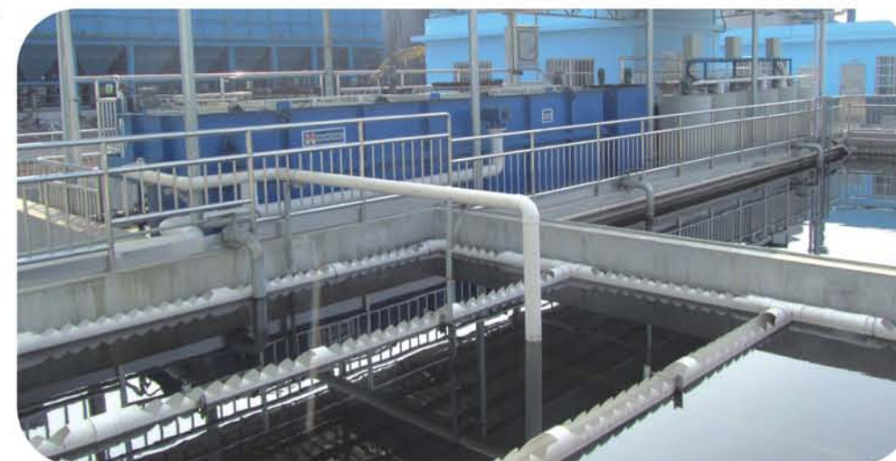
Casting center wastewater treatment station
