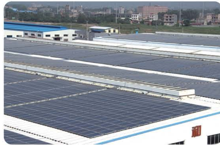
PV modules are neatly laid on the roof of the workshop
