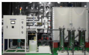
Water Recycling and Filtration System Installed at the Cable Tunnel of the Namcheongju Office
