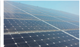
PV Power Plant at the kt Gwangneung Transmission Facility
