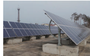
PV Power Plant at the kt Gwangju Transmission Facility
