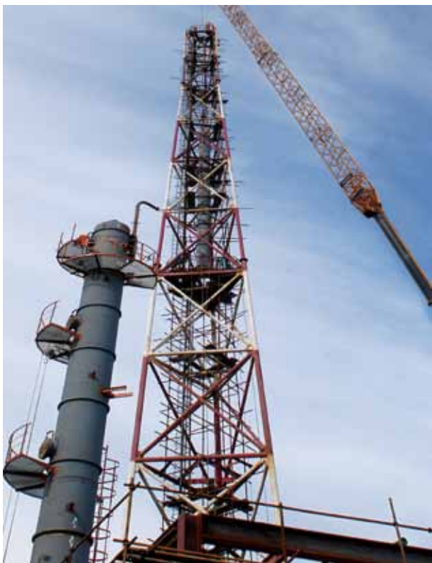
Installing a new funnel in Sinopec Cangzhou Refinery, which was revamped during the overhaul for better tail gas treatment. Environment protection units were added or replaced to the existing sulfur recovering facilities. All H 2 S can be recovered and reused, which brings both economic and environmental benefits
