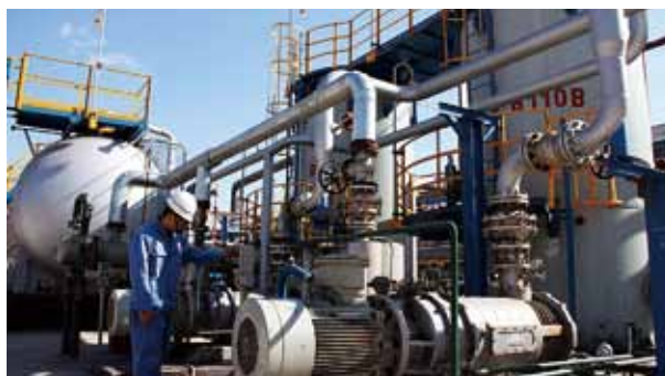
A technician from Sinopec Yanshan Company is checking pressure swing tail gas adsorption facility with a PP recovering capacity of 1,630 tpa
