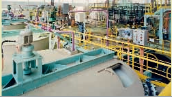
Liquid effluent treatment unit
