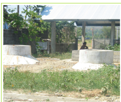
Biogas digesters for piggeries project in Laoag City
