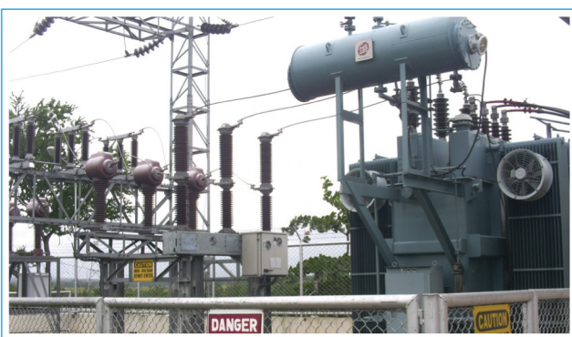
Power Sub-Station project in Bataan
