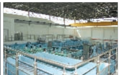
Water & Sewage Treatment Demonstration Plant
