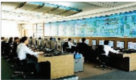
World's Largest Metropolitan Integrated Operations Center
