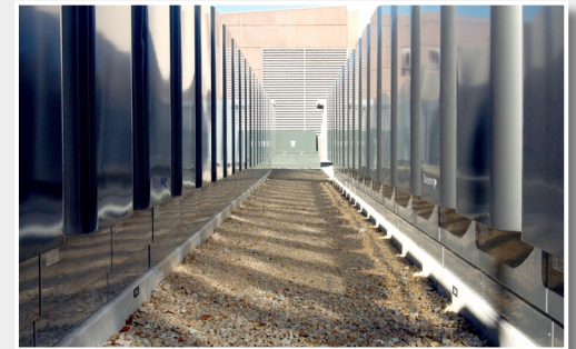
The new data center is one of the first to use cleaner energy fuel cells as its primary power source.
