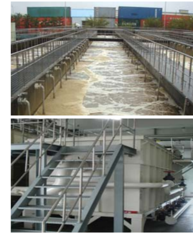
• Dissolved Air Flotation Facility 1 Aeration Tank 2
