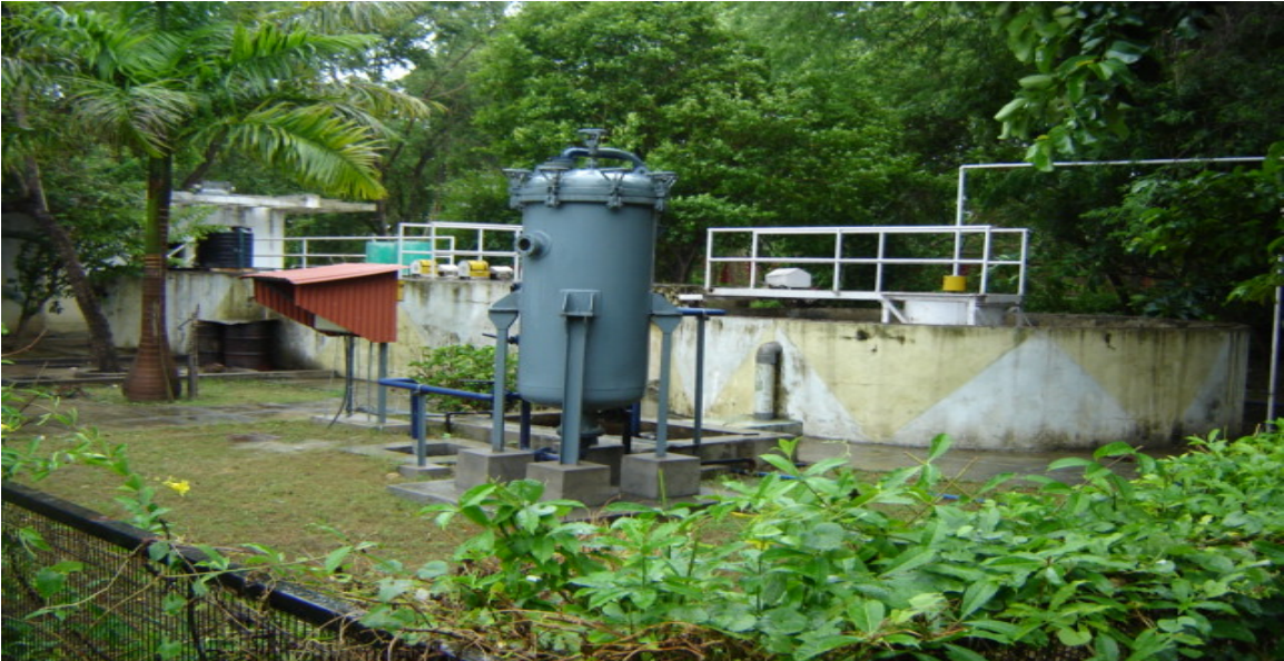
Fig.: Effluent Treatment Plant Upgradation at Lucknow Plant
