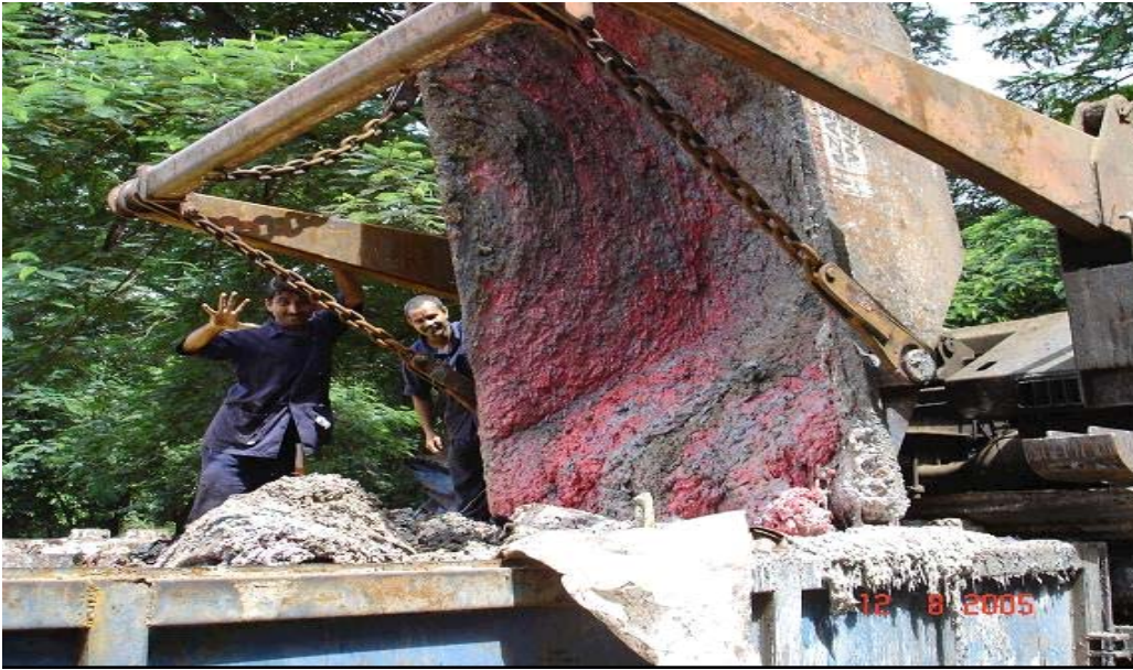
Photo: Paint sludge (hazardous waste) from our dumper trucks being directly transferred into the custom built containers of CHWTSDF
