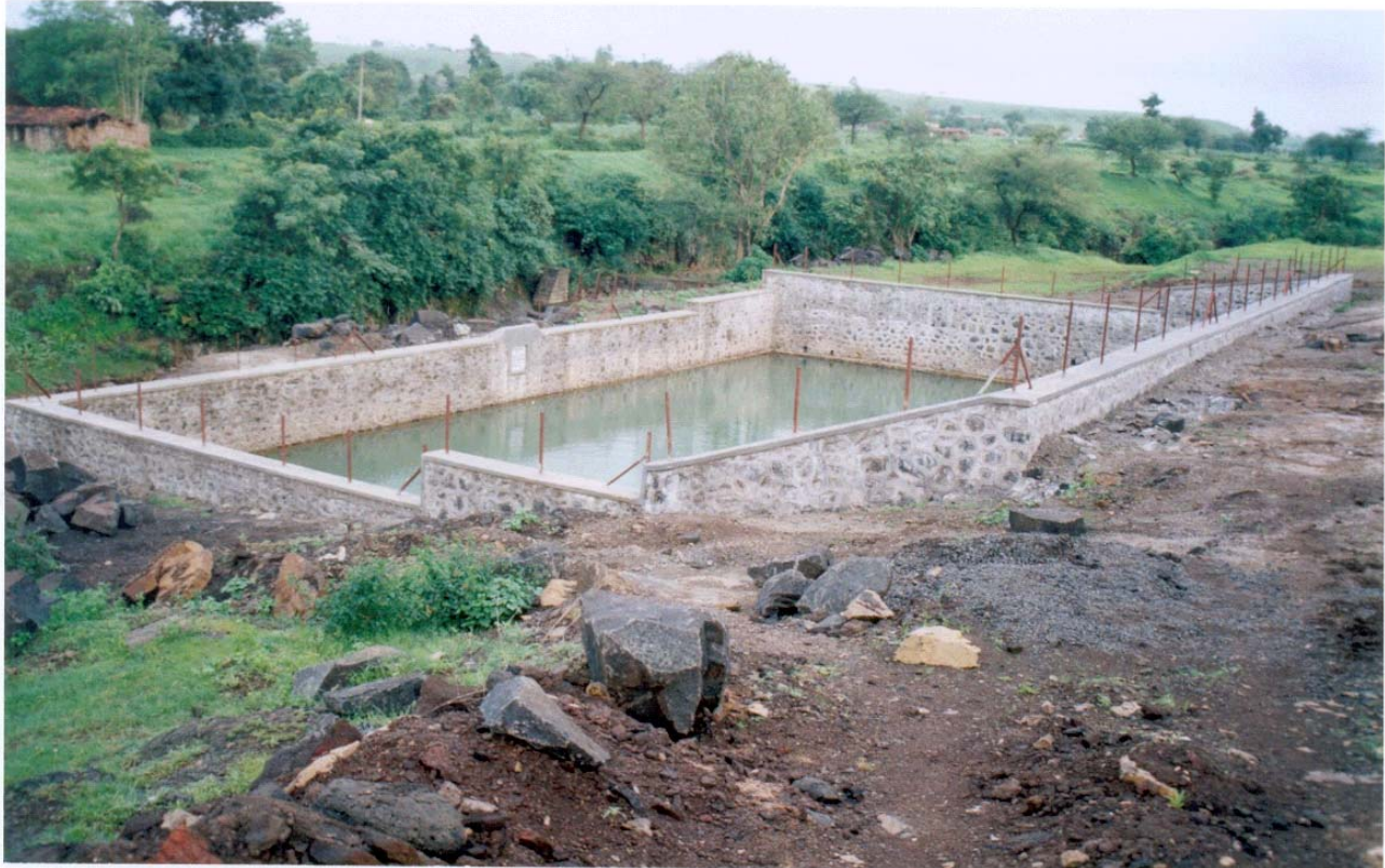
Fig: Rain Water Harvesting at Pune Plant
