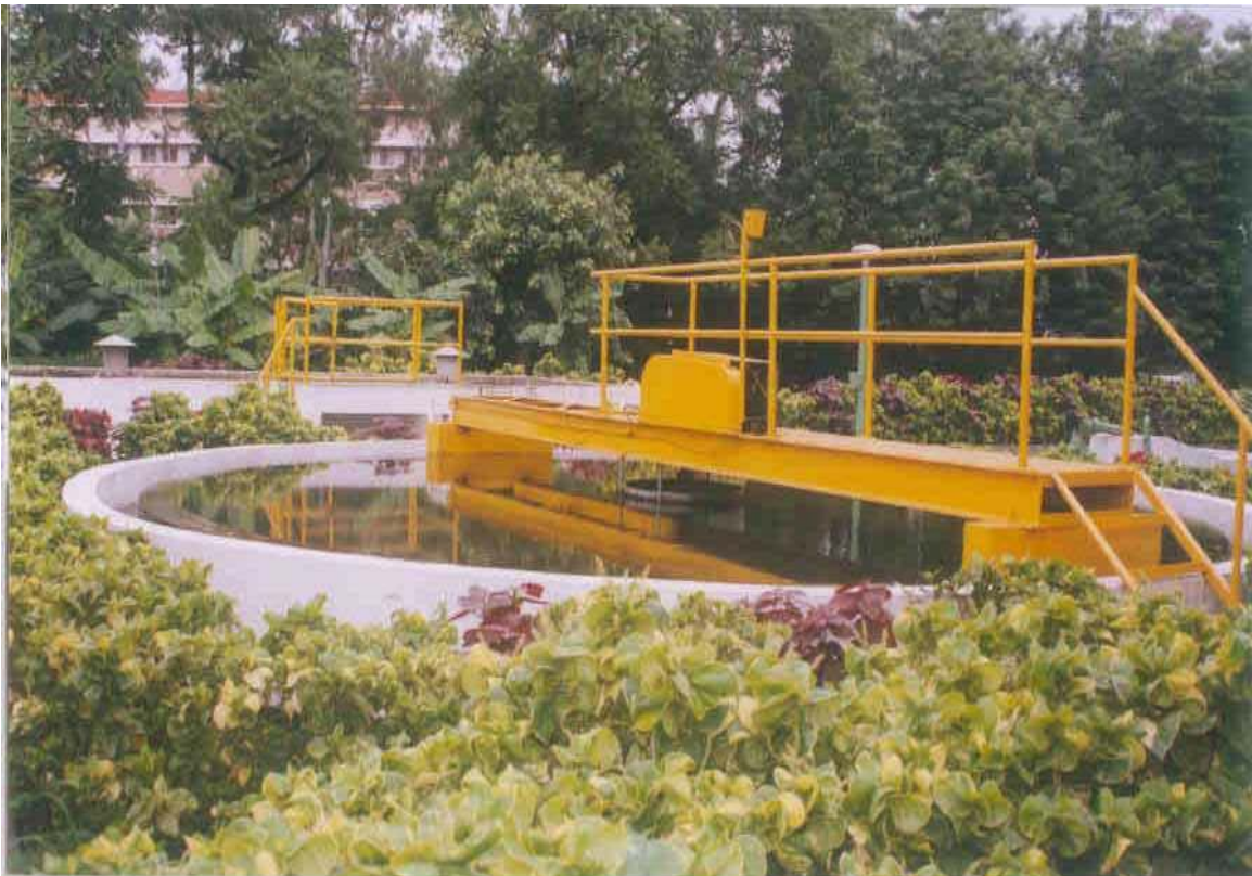
Fig.: Effluent Treatment Plant at Pune
