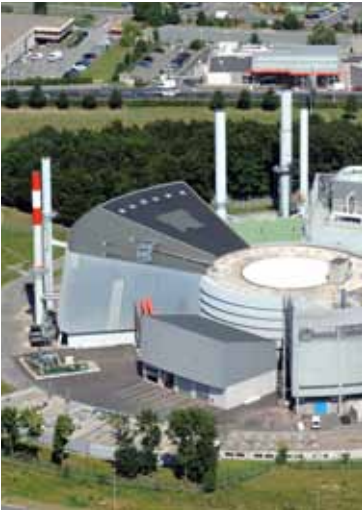
Two wood-fired boilers at Paris-Charles de Gaulle provide 25% of the heating needed at the airport without releasing fossil-fuel CO2 emissions.
