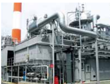
Hikari Plant: Boiler facility
