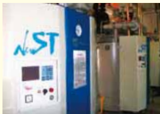
Tianjin Takeda Pharmaceuticals Plant: A newly installed boiler at the plant runs on city gas
