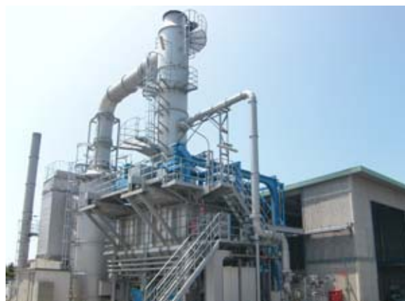
Burnable waste at the Hikari Plant is incinerated in a state-of-the-art gasification facility fully equipped to counter dioxin releases
