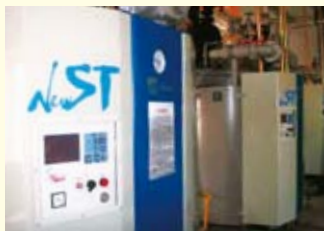
Tianjin Takeda Pharmaceuticals Plant: A newly installed boiler at the plant runs on city gas
