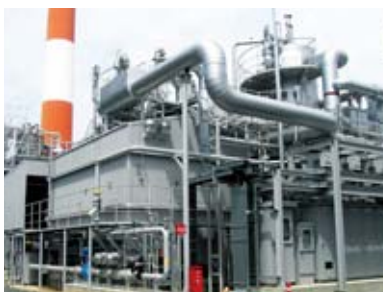
Hikari Plant: Boiler facility
