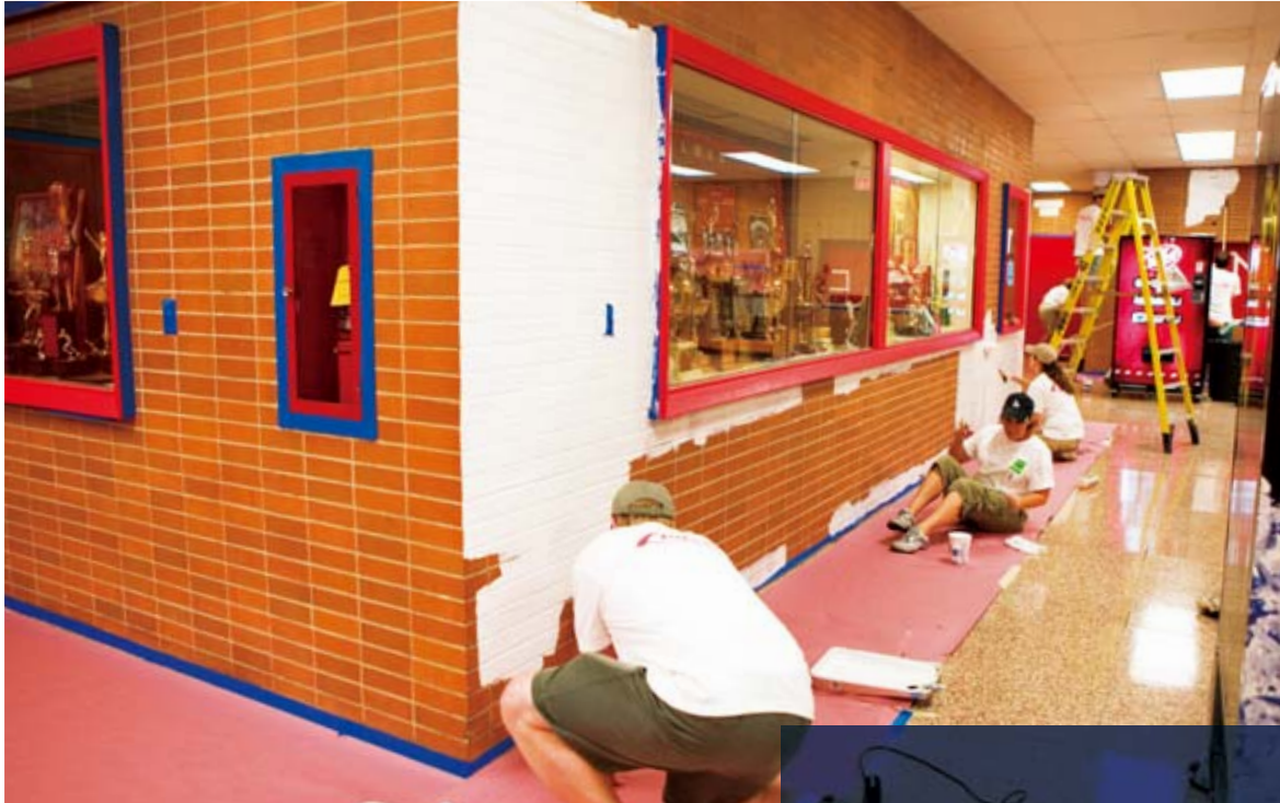
TPNA employees apply a new coat of paint to brighten up a wall
