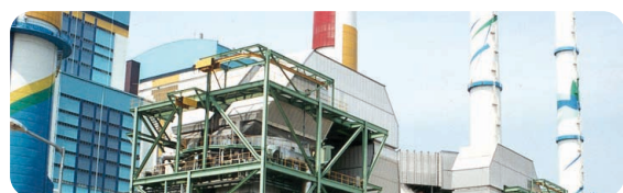
▲ Flue Gas Desulfurization(FGD) Facilities
