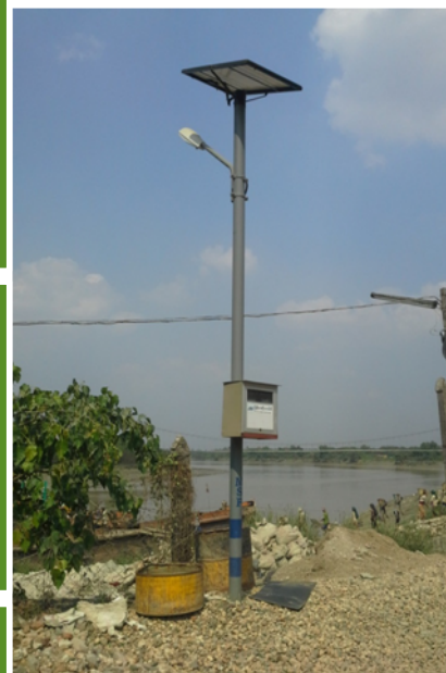
Solar Street Lamps are used in our factories at Shwe Pyi Thar Township, Tharkayta Township and Thingangu Township, Yangon
