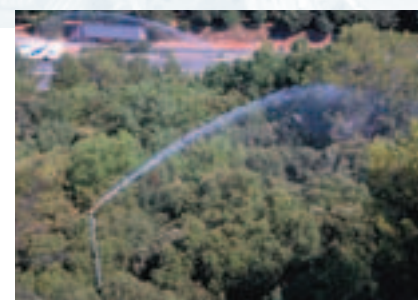
Automatic sprinkler system, known as SPACI, in a motorway area.
