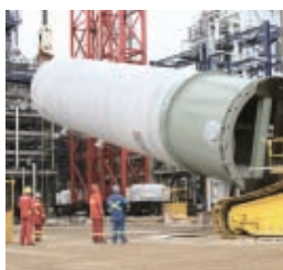
A reactor vessel is installed at the Edmonton refinery as part of the diesel desulphurization project. The reactor is a key piece of equipment that will enable Petro-Canada to meet federal regulations requiring diesel fuels to contain no more than 15 parts per million in sulphur in 2006.
