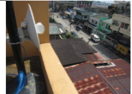
Communication equipment in Tacloban.
