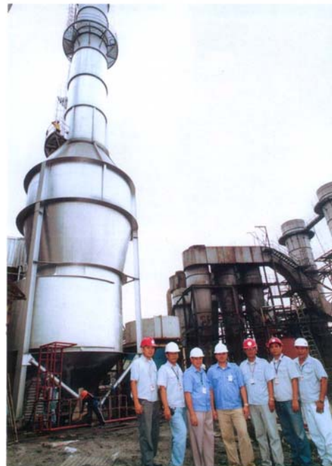
Wet scrubber system retrofitted into one of the boilers of the CADPI plant, with the project team.
