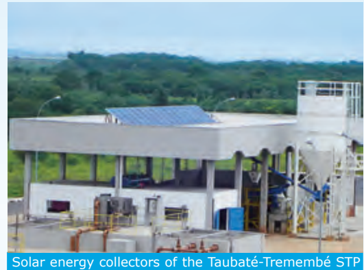
Solar energy collectors of the Taubaté-Tremembé STP
