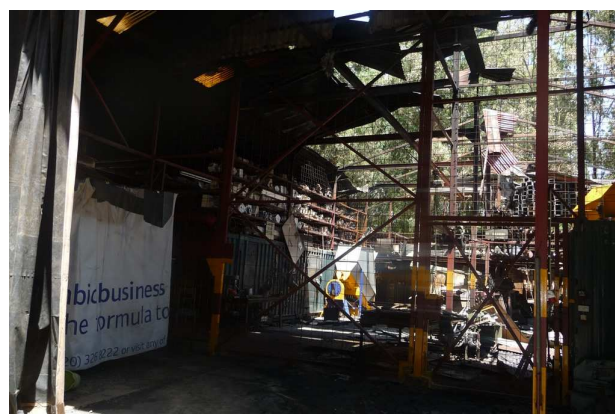
FIGURE 2: BURNT DOWN WORKSHOP
