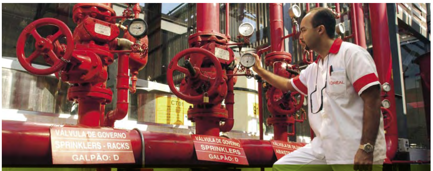
► Inspection of our fire sprinkler system in our Rio de Janeiro (Brazil) factory.
