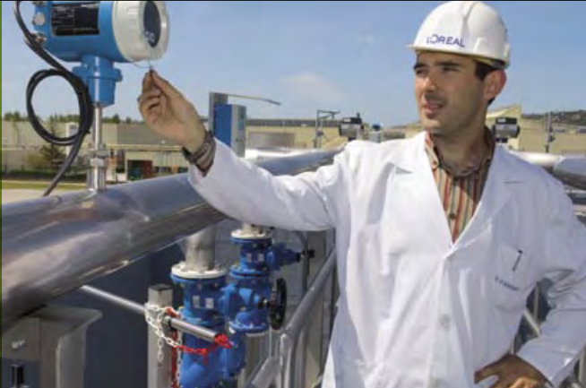
► An oxygen meter reading at our Burgos (Spain) wastewater treatment site.
