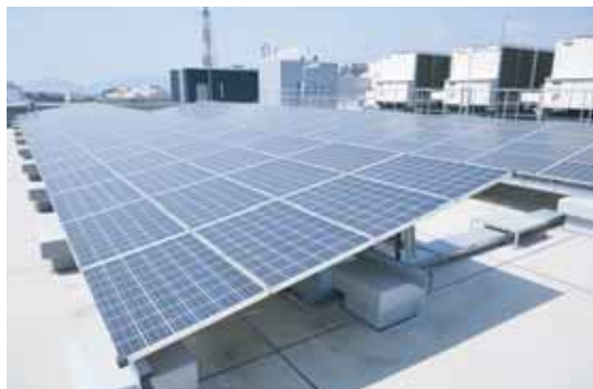
Solar Power Generation Facilities at Hikari Plant
