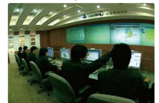
• CleanSYS Control Center at the Capital Area
