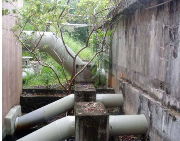
Drain connected to pipes to a tank outside
