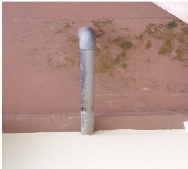
Pipes accumulating rain water directed to a tank underground
