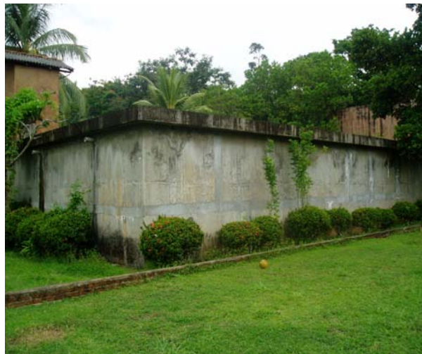
The tank in which water is stored for re-use
