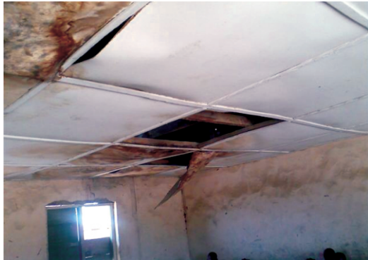
Interior of classrooms at St. Mark's School Awoyaya, before CAP Plc's intervention.
