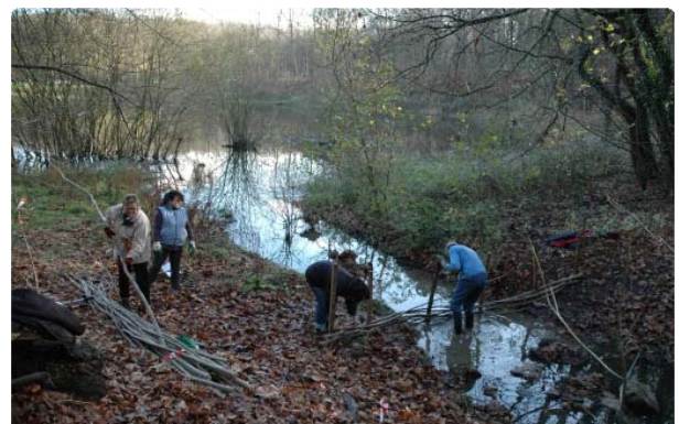
Building one of the dams that help prevent leaves filling the pond
