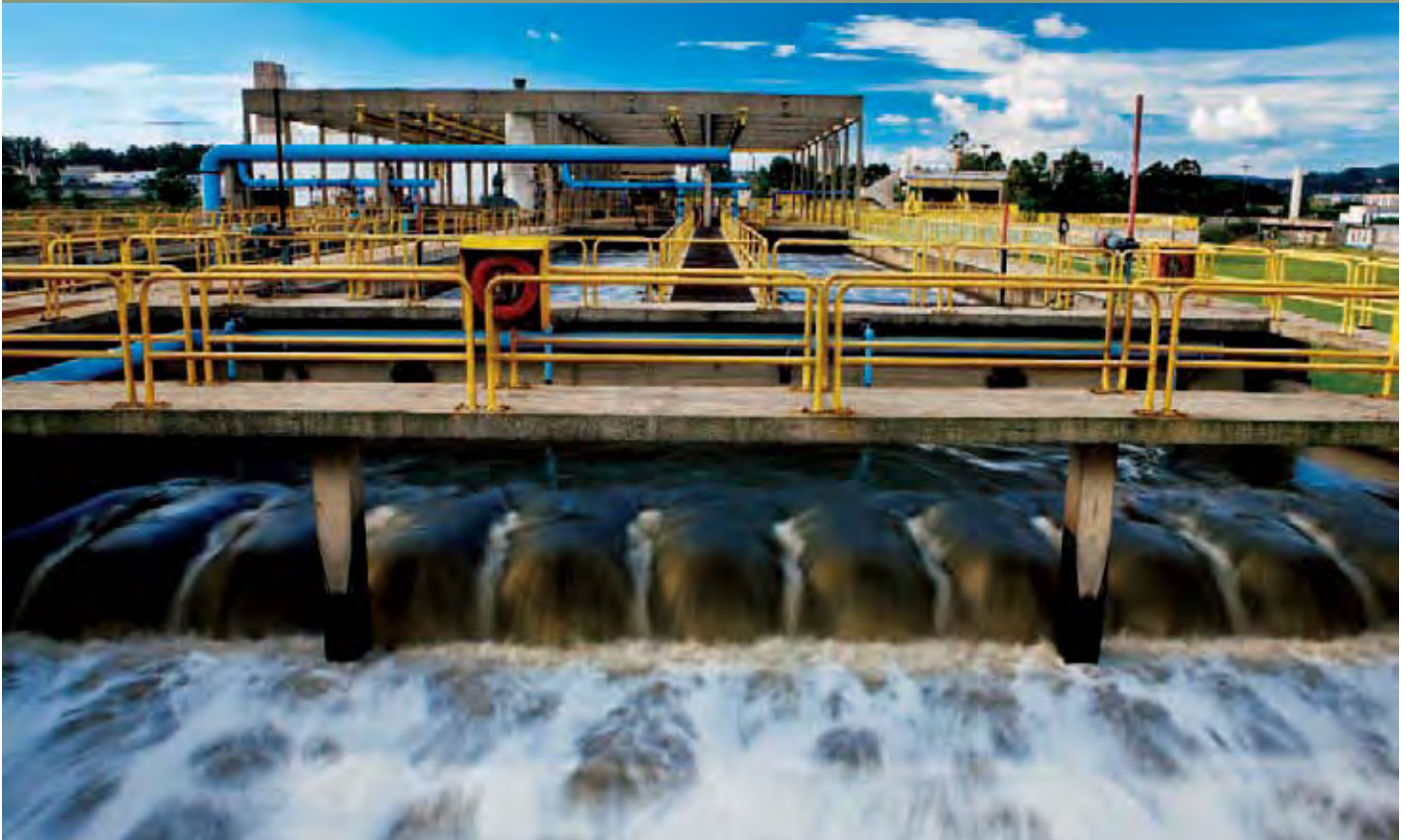
Barueri Sewage Treatment
