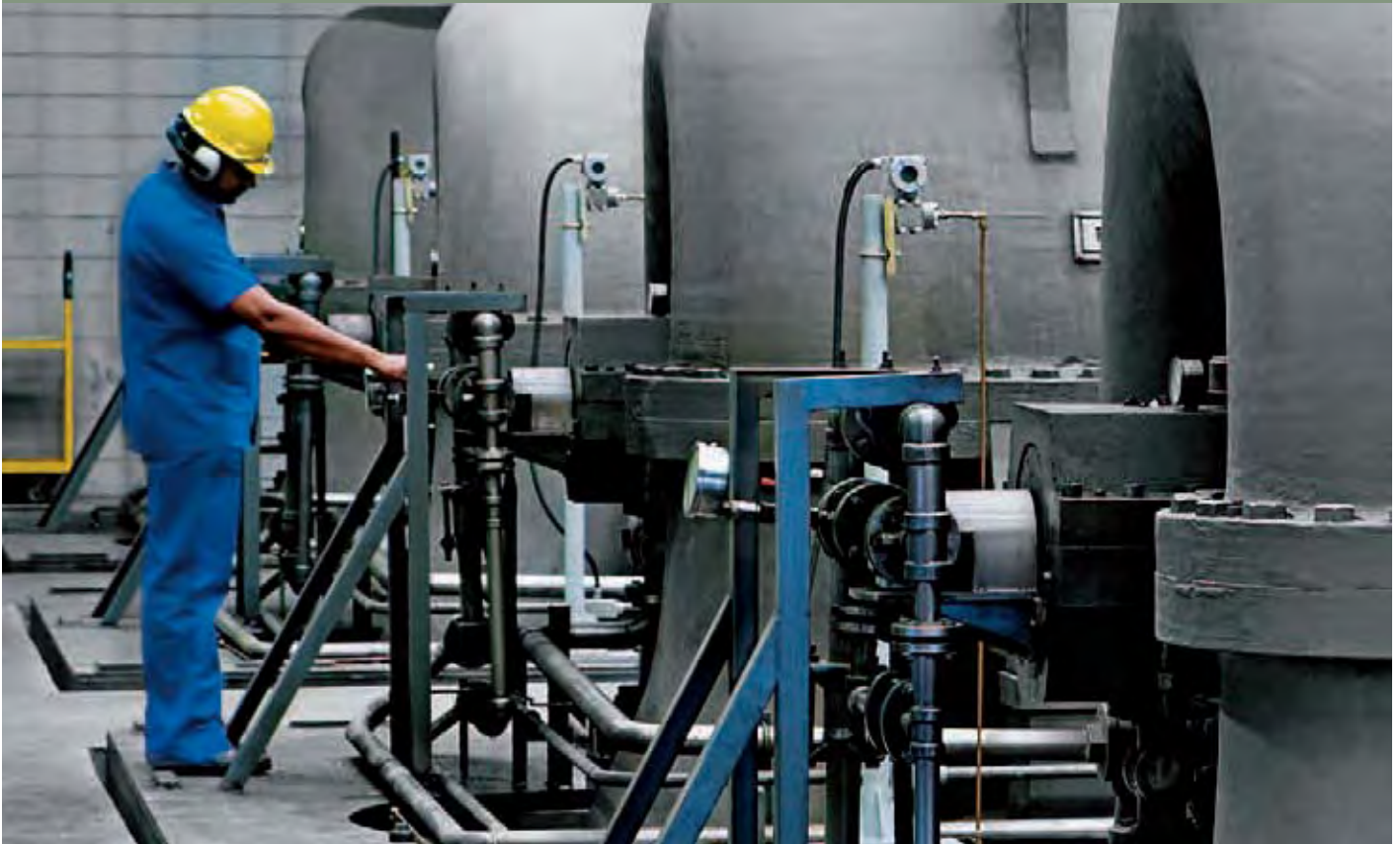
Barueri Sewage Treatment Station.
