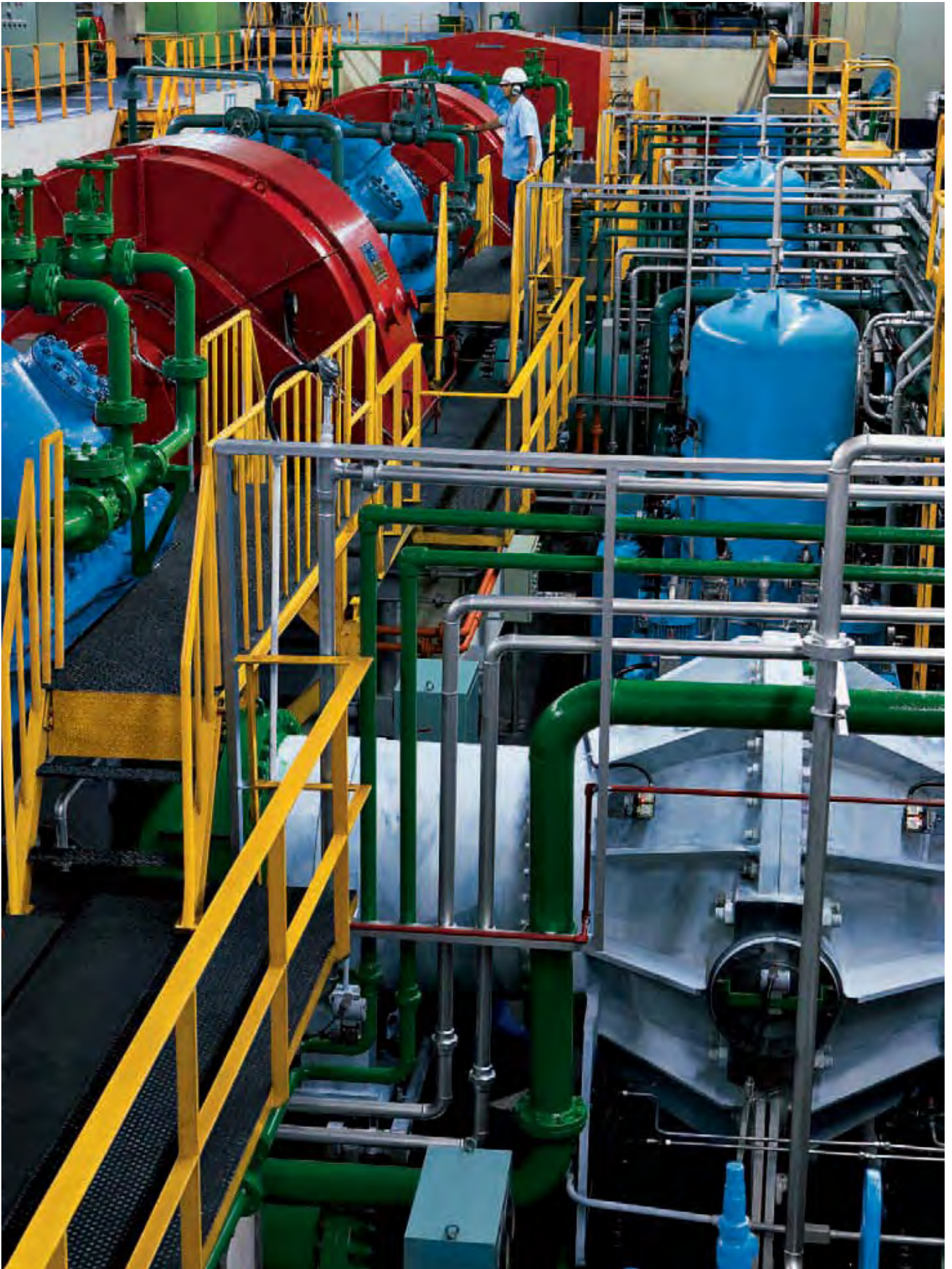
Santa Inês Lift Station.
