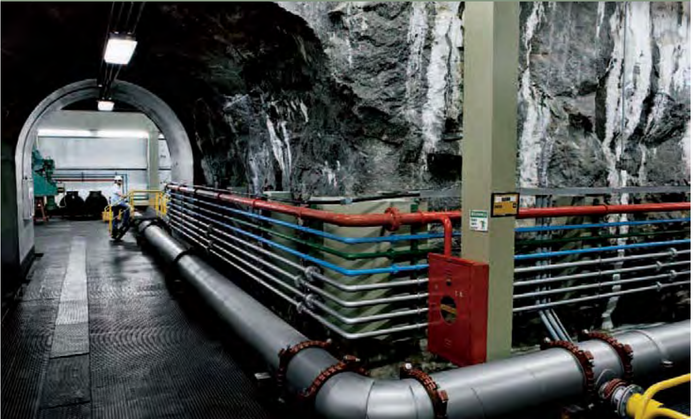
Santa Inês Lift Station.
