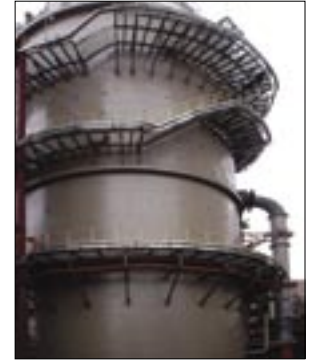
2# line desulfurizing tower
