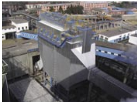
The flue gas emission concentration is less than 30mg/m after the dust removal modification of thermal-electric No. 1 boiler
