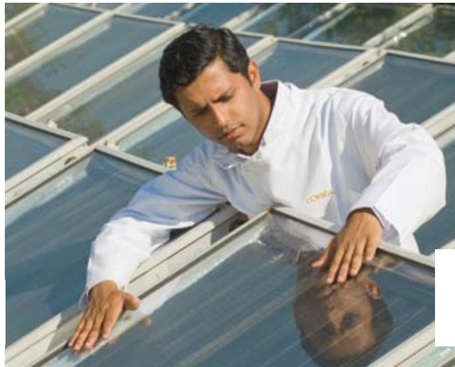
Solar water heating panels, Pune factory (India).
