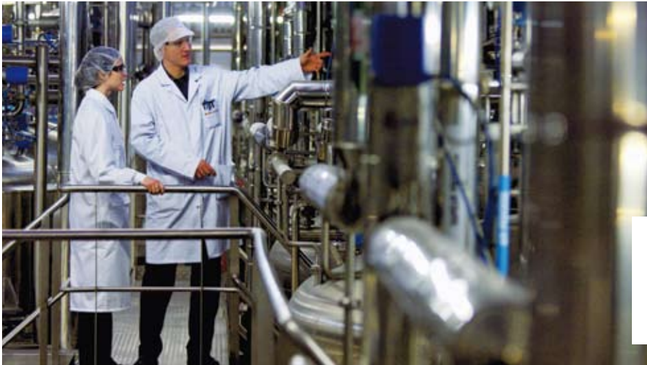
Our factory in Rambouillet (France) has installed a system to recover waste heat. This has resulted in a 23% reduction in natural gas use per year, with an 8% reduction in electricity use.
